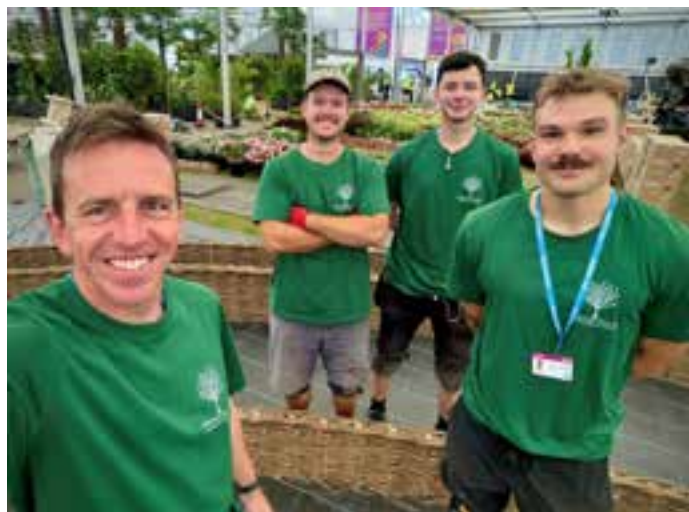
Left to right: Chris Webster, Charlie Temple, Jake Whiting and Josh Hart during the willow rose bed construction in the RHS Chelsea Grand Pavillion
